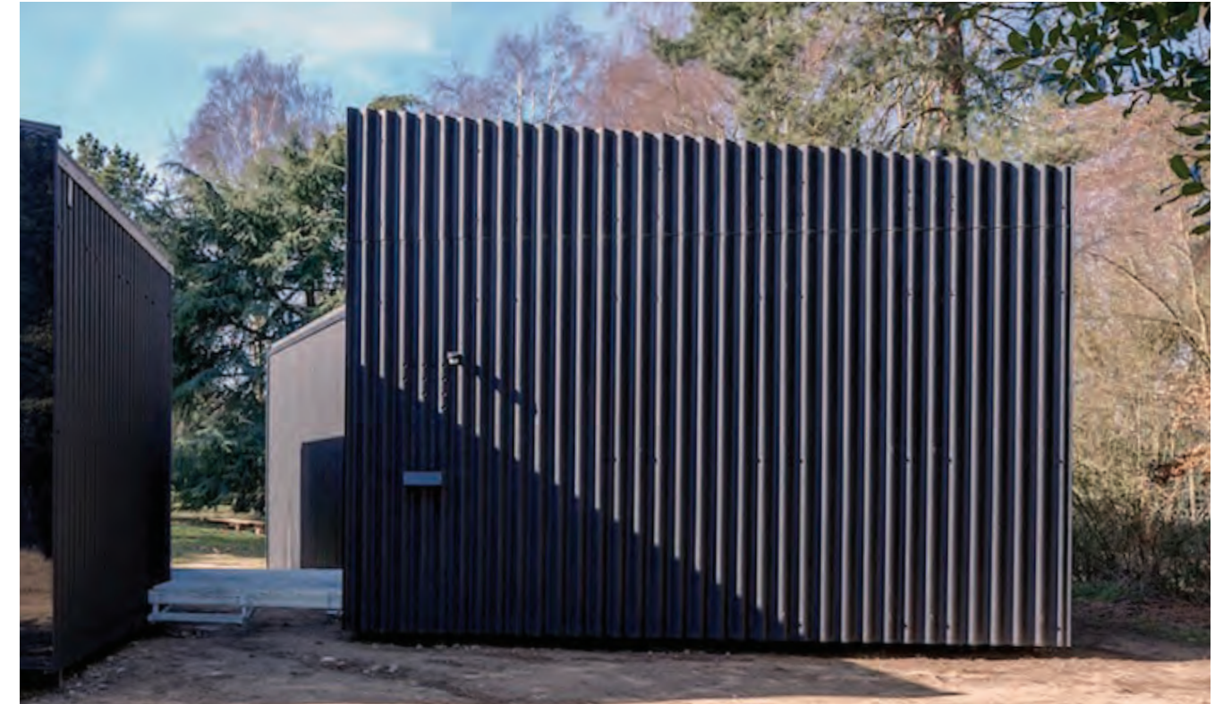
Figure 11: Fibre Cement Example 1
