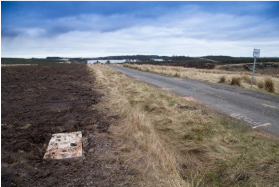
Plate 2 Example below ground link box following reinstatement (Source: Rey Wind Farm, Vattenfall Wind Power Ltd.)
