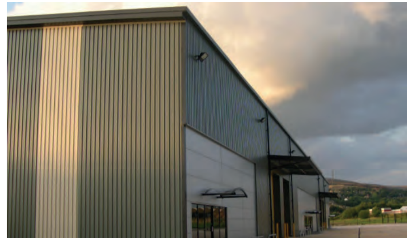
Figure 12: Fibre Cement Example 2
